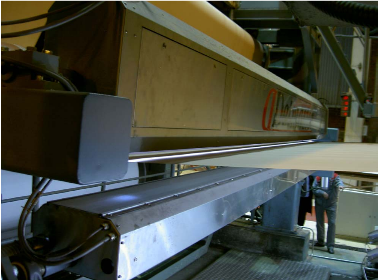
Detmaster 5200 PRT system installed at Stora Enso Imatra mills' board machine No. 5.
